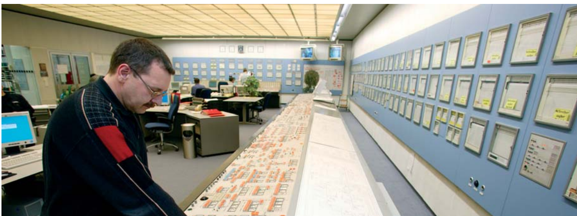
All the power plant systems and processes are controlled and monitored from the central control rooms of the two units A and B.
