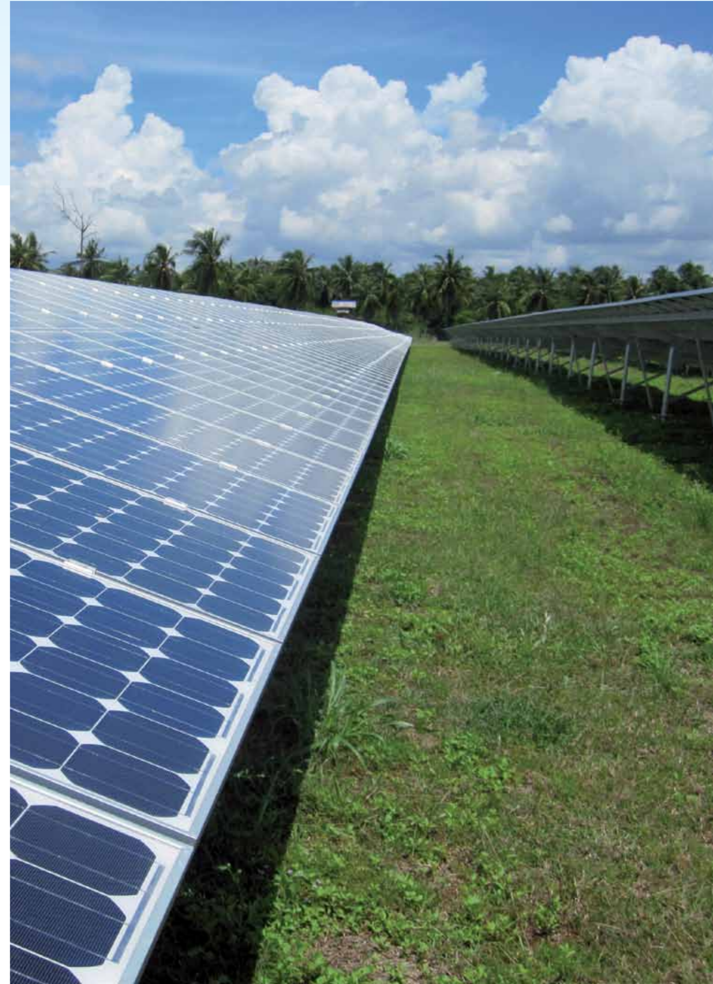
Chonburi Solar Park, Thailand
