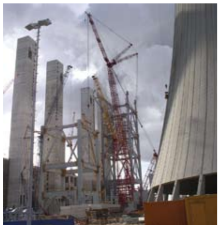
Site as of 5 March 2008. The picture shows the four stair towers, two per unit and, in the centre of the picture, boiler structural steel for unit F (right), where the October accident occurred, and for unit G (left)
