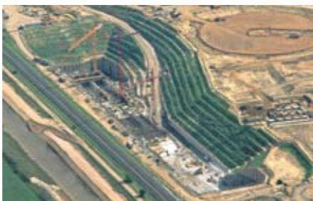
The excavation for the underground bunker (Sept 2006), up to 43 m deep in parts
