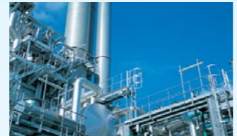
RWE operates and maintains the cogeneration plant at Bridgewater Paper, UK
