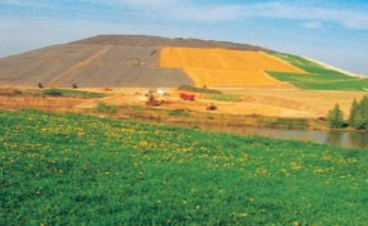
Beerwalde – rehabilitation work in progress on waste rock dump of a uranium mine in Germany
