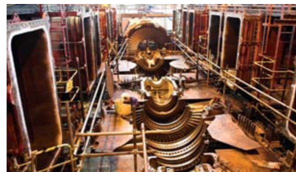
Overhaul of Didcot steam turbine Right: CCGT rotor blade inspections prior to lowering rotor into turbine casing
