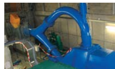
New Pelton Unit at River E
