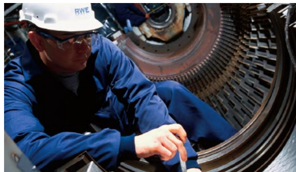
Turbine bearing check
