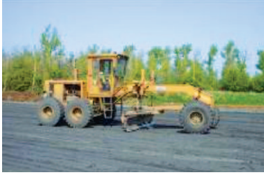
A wheeled grader used to spread thin layers of ash on site
