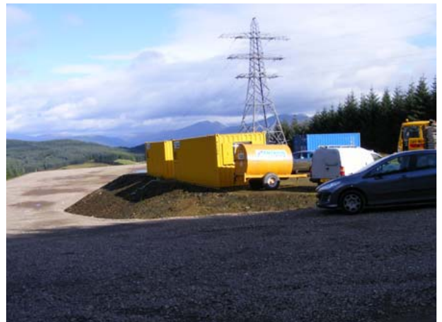
October 2008, Substation platform.
