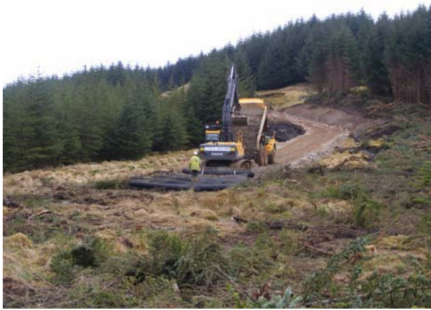
March 2009, Floating in a road.
