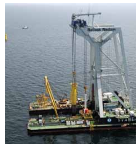
(Photos above) HLV Svanen will install the foundations of Rhyl Flats Offshore Wind Farm.
