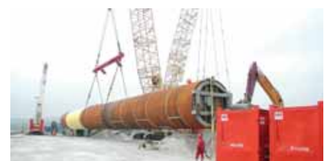
(Photos above) A monopile is delivered to Mostyn Docks during construction of North Hoyle Offshore Wind Farm.
