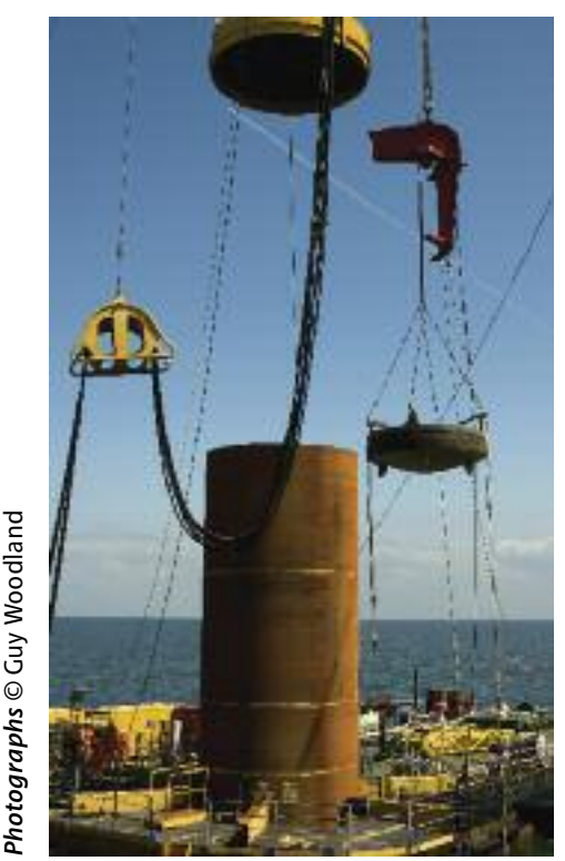
The pile hammer is moved into position ready to sink the monopile into the seabed.
