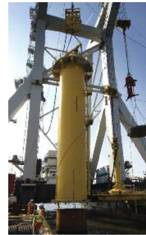
A transition piece is lifted on top of the newly sunk pile.
