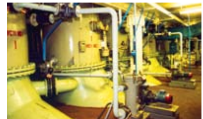
Condenser tube cleaning system
