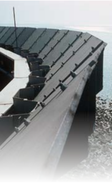
Top: Sheet pile wall with wave deflector. On the sea side, the sheet pile wall extends to a height of 11 metres. Nothing can enter from the outside, apart from rain and spray. And nothing can escape to the outside, not even rain water.
