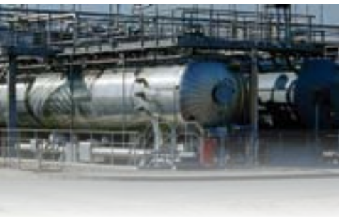
Top: The entire operations of the Land Station are constantly monitored by specialist personnel from the control station.
