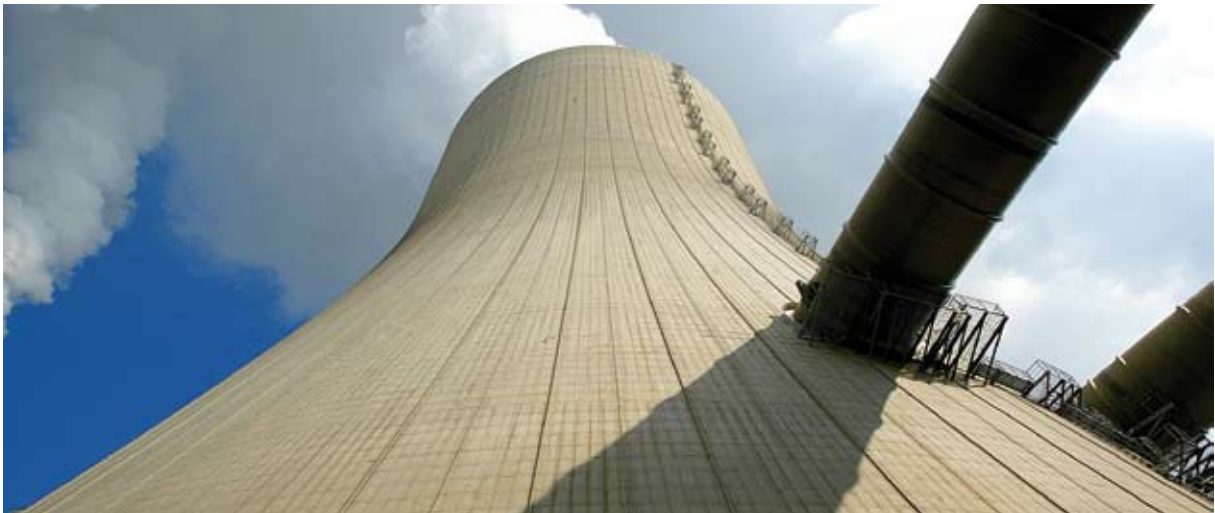
Fig. 1: Outside view of the BoA cooling tower and the flue-gas ducts in Niederaussem
