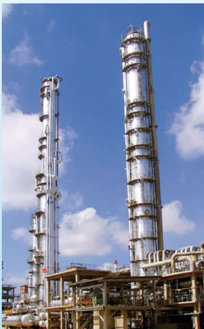
Plant for chemical scrubbing
