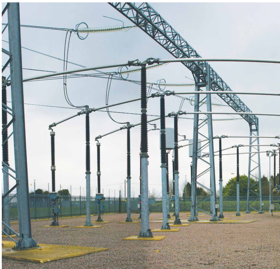
This photograph shows what part of an electricity substation could look like
