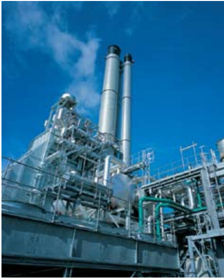
One of npower Cogen's dedicated CHP plants
