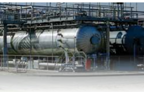
Top: The entire operations of the Land Station are constantly monitored by specialist personnel from the control station.
