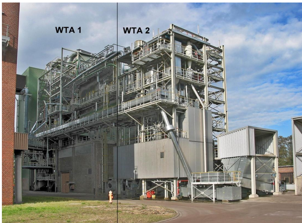
Fig. 9: Photo of the WTA 1 plant (left part) and WTA 2 plant (right part) at Frechen
