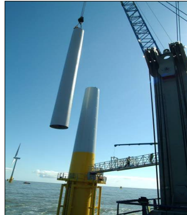
Figure 4: Turbine tower construction at the now operational RWE npower renewables Rhyl Flats offshore wind farm, North Wales
