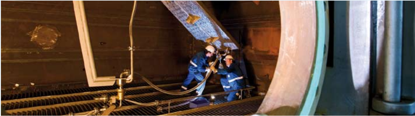
A look into the dryer of the WTA prototype plant at Niederaussem
