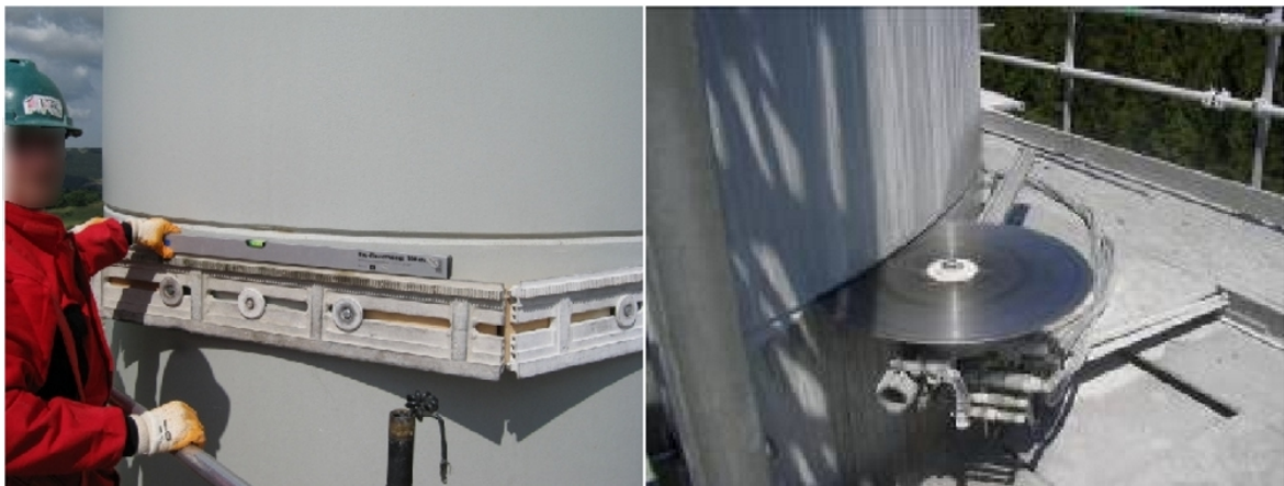
Fig. 9: Guide rail for the concrete-wall saw bolted to the tower segment (left); concrete wall saw (right)
