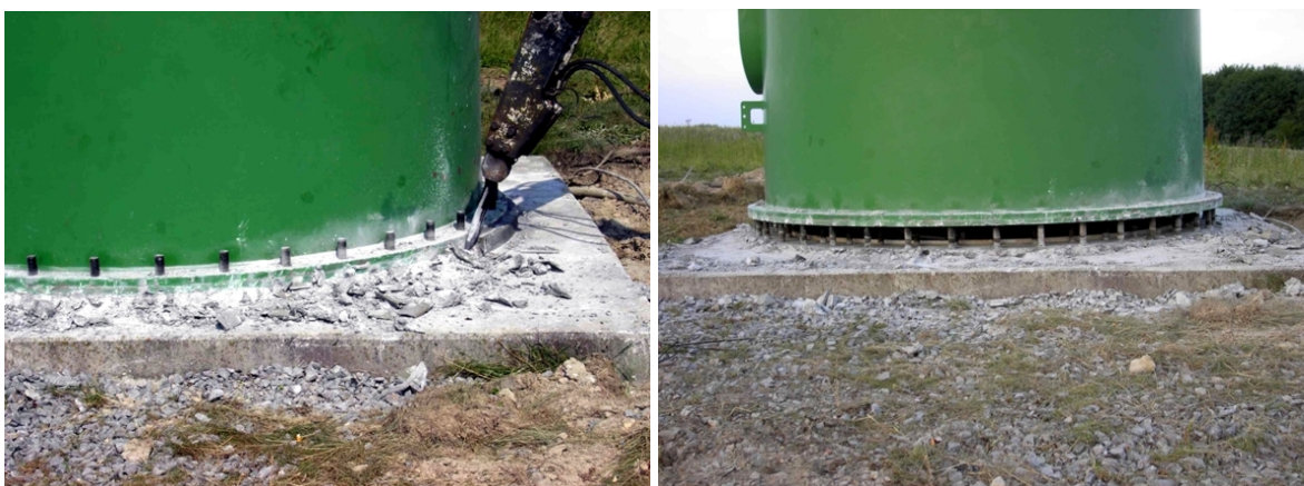
Fig. 17: Separating and lifting the lowermost steel section on a tower with a foundation basket
