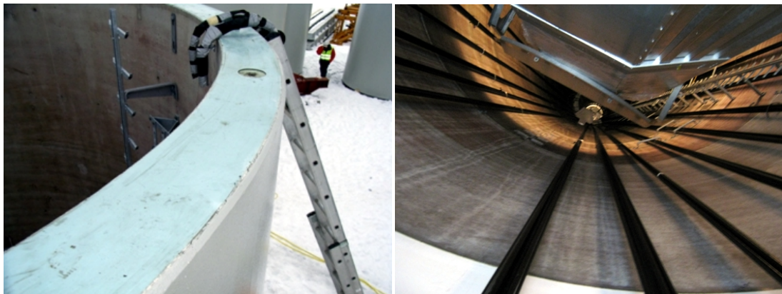
Fig. 7: Horizontal joint levelled (left); prestressing tendons on the inside of the tower (right)
