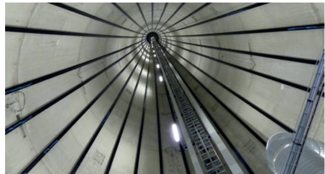
Figure 4.5-2 : View inside the power plant with 143 m hub height. Photo: LUBW
