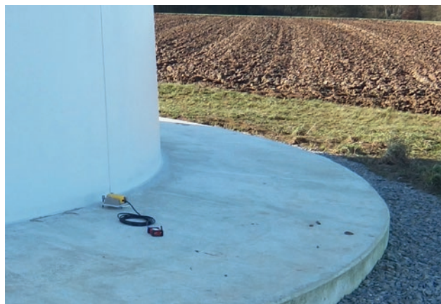
Figure 4.8-1: Vibration measurement point MP A at the tower foundation of WT 5. Photo: Wölfel company
