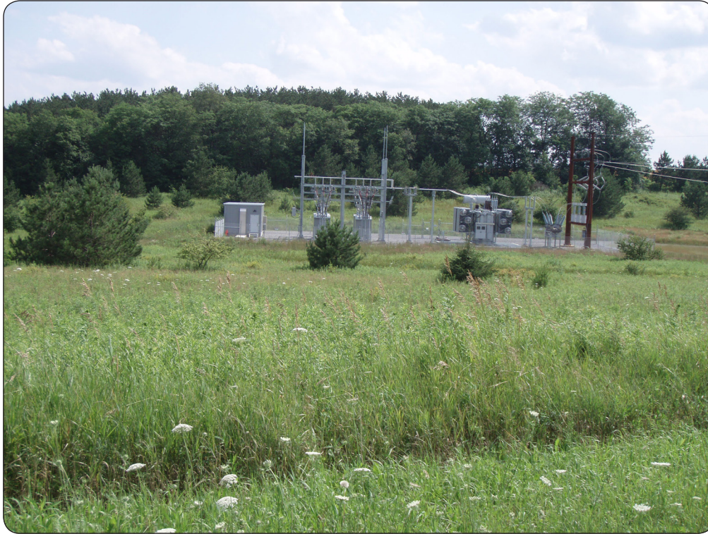
Photo 1: Cohocton Wind Farm Collection Substation
