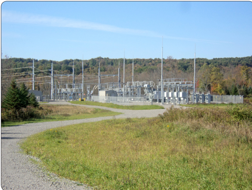
Photo 2: Hardscable Wind Power Project Point of Interconnect (POI) Substation
