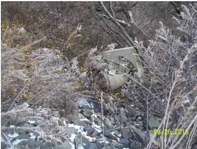
FAILURE OF A CULVERT CONCRETE END SECTION DUE TO WASHOUT
