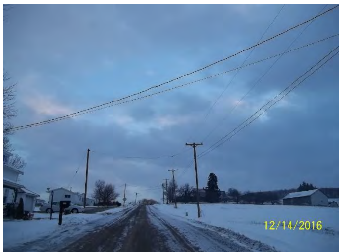
SEVERAL LOCATIONS OF LOW WIRES NEAR NY 21
