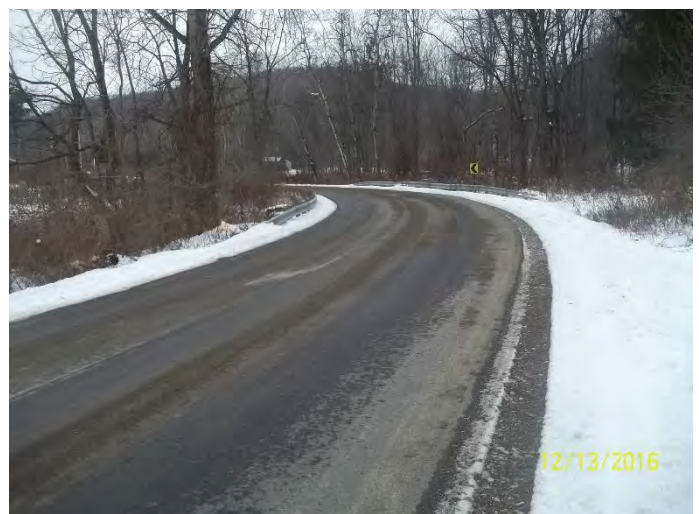
SHARP CURVE OVER CULVERT WITH RAILING
