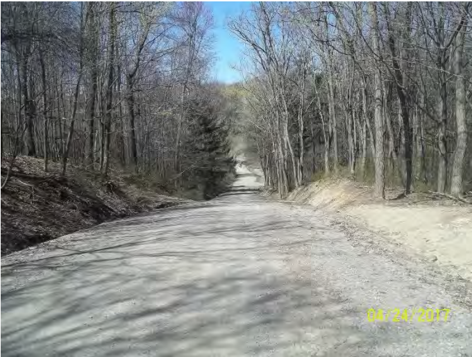
SEGMENT WITH STEEP GRADE WITH DEEP DITCHES 0.2 MILES EAST OF DUTCH RD
