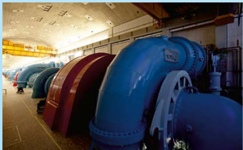
Turbine hall of the Vianden pumped-storage power plant
